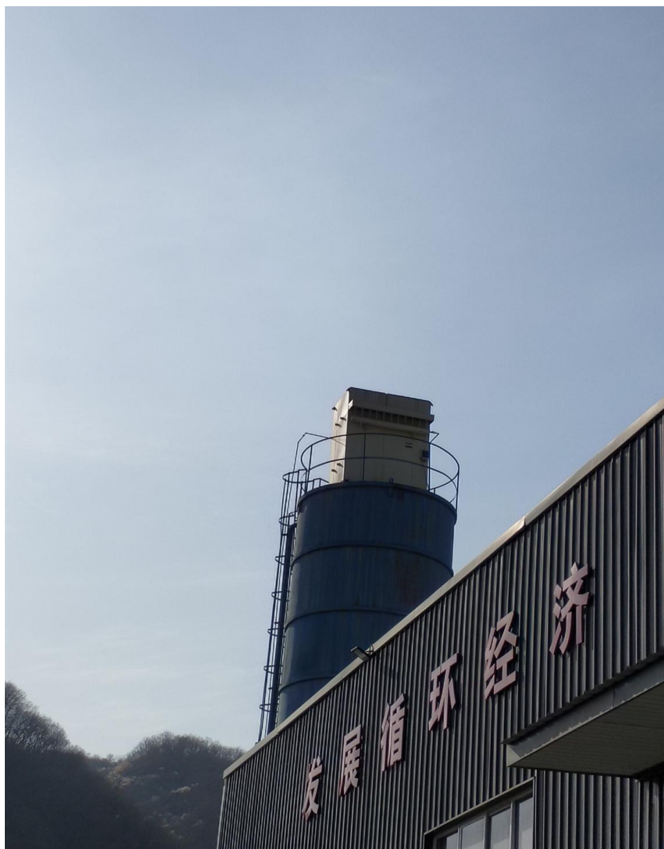
储灰仓仓顶除尘设备
